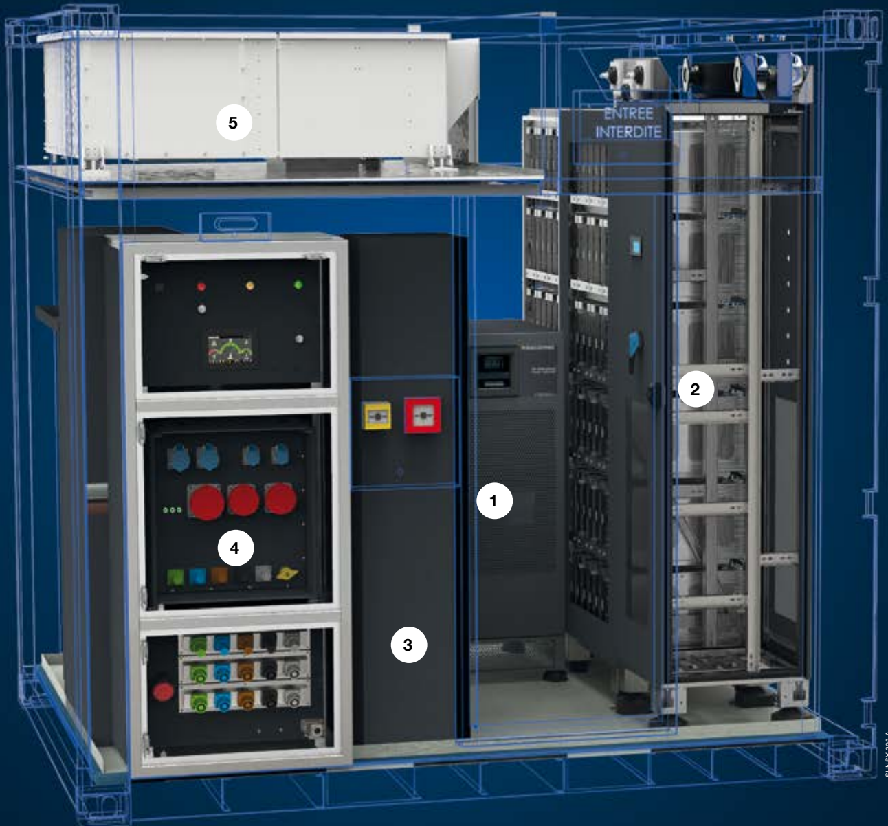
SUNSYS Mobile 200kVA/330 kWh built into a 10' ISO High Cube container
